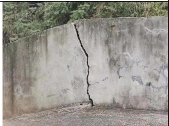
溢洪道边墙破损
